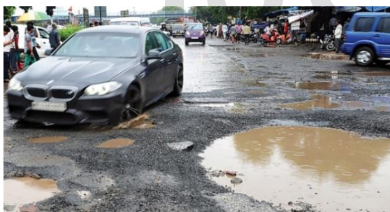
Fig2:potholes in roads
