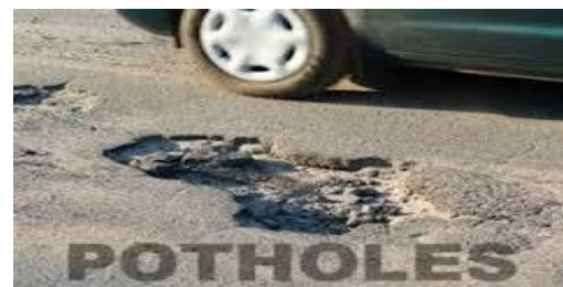
Fig.1: road condition with potholes.
